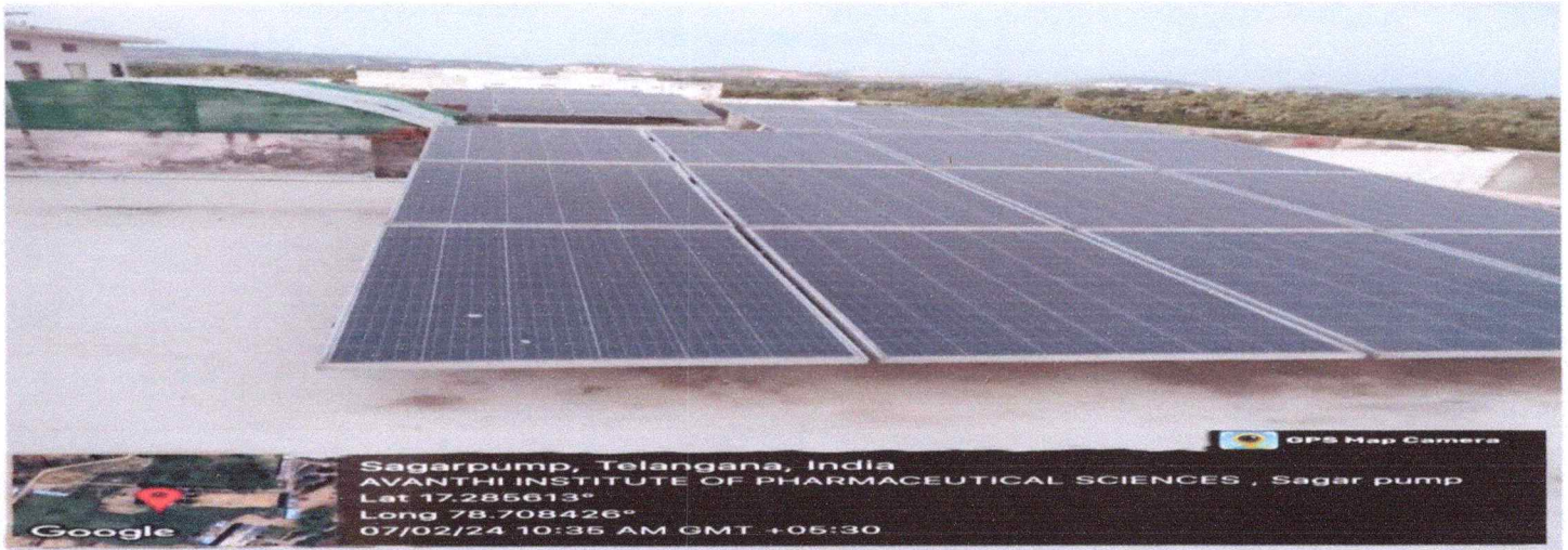
FIG: 6 Installed solar panels that consist the capacity of 60 KW Each
