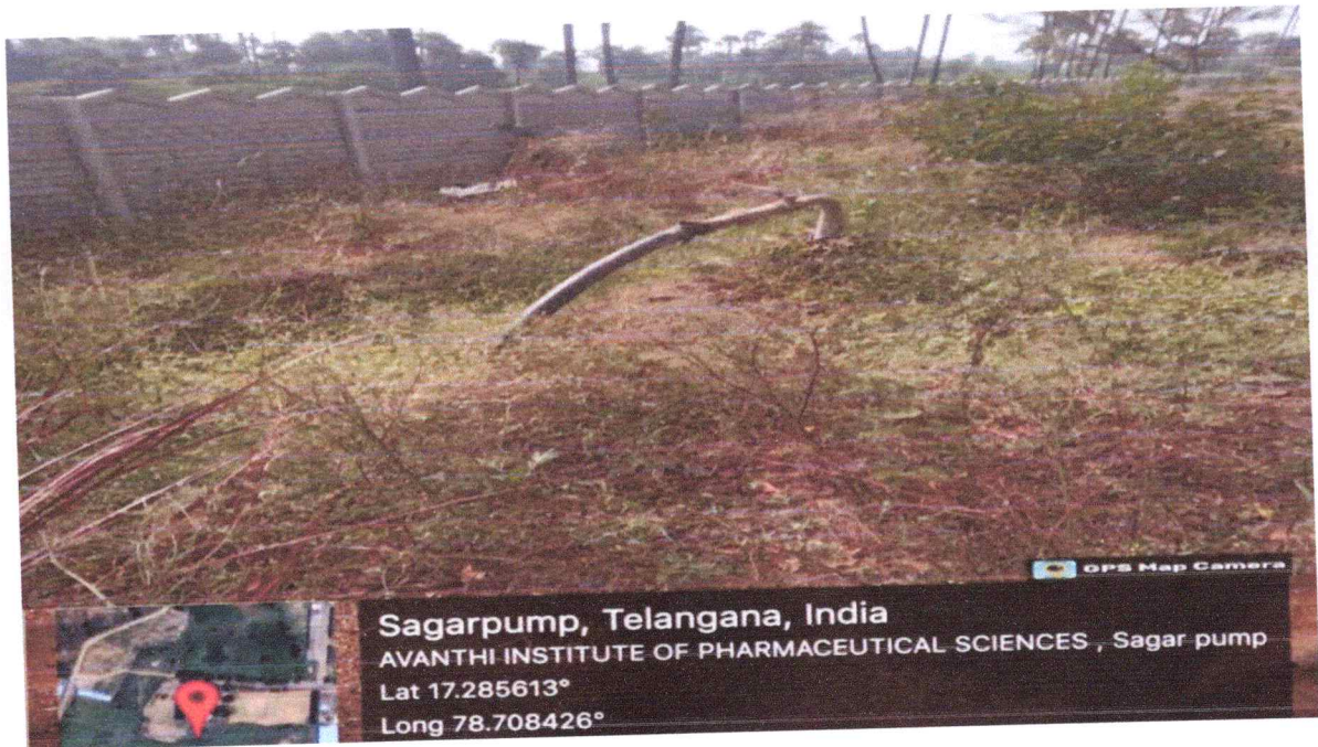
FIG: 7HP Motor capacity was installed near the Pharmacy block
