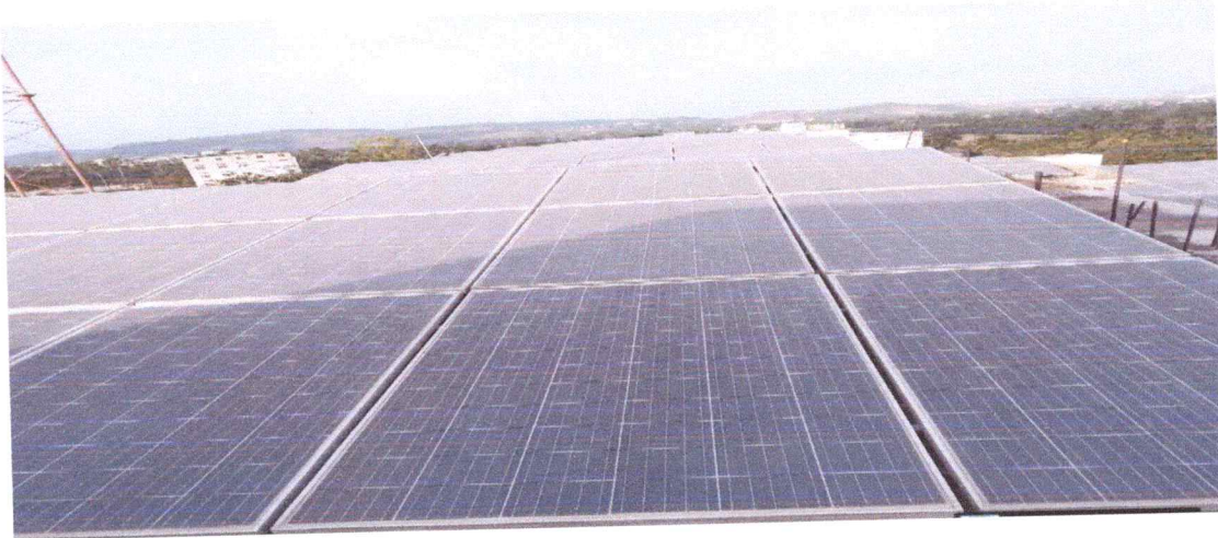
FIG: 6 Installed solar panels that consist the capacity of 60 KW Each
